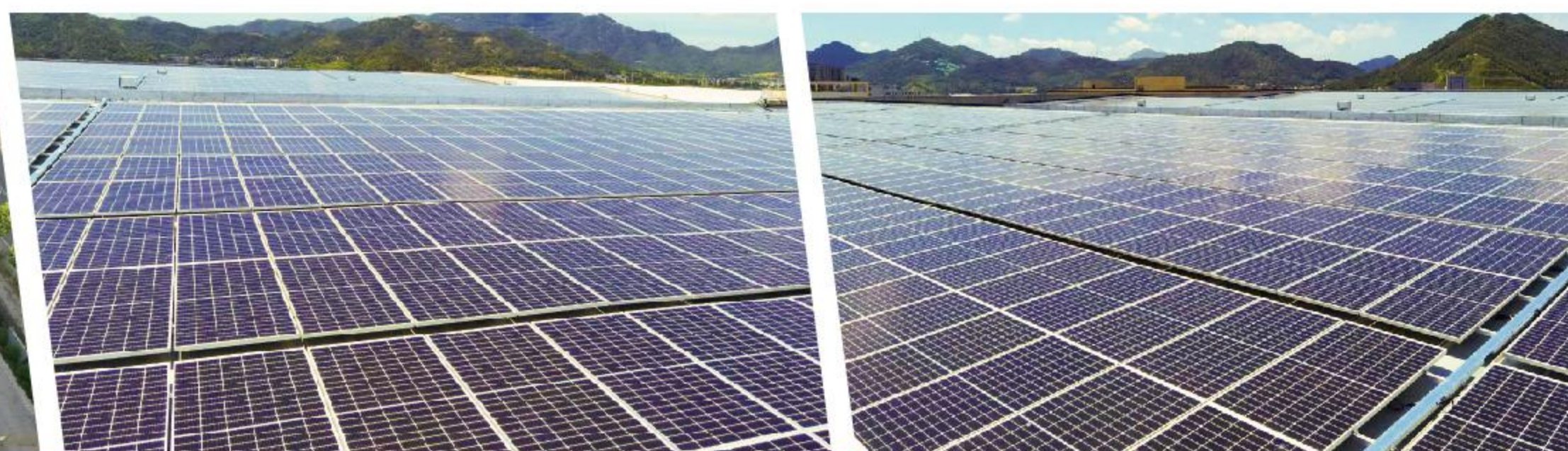
▶ Ningbo Xiangshan 5.7 MWp project
