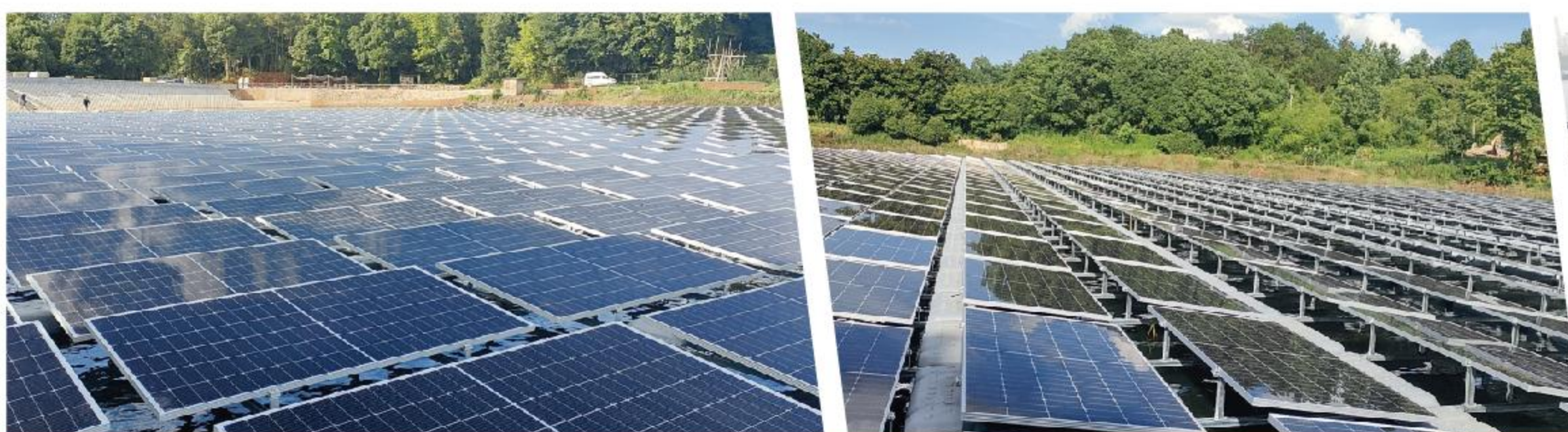
▶ Shaoxing 2MWp surface power station
